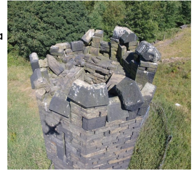
Walker Pit Tower damage Photo: Courtesy of David Glover
